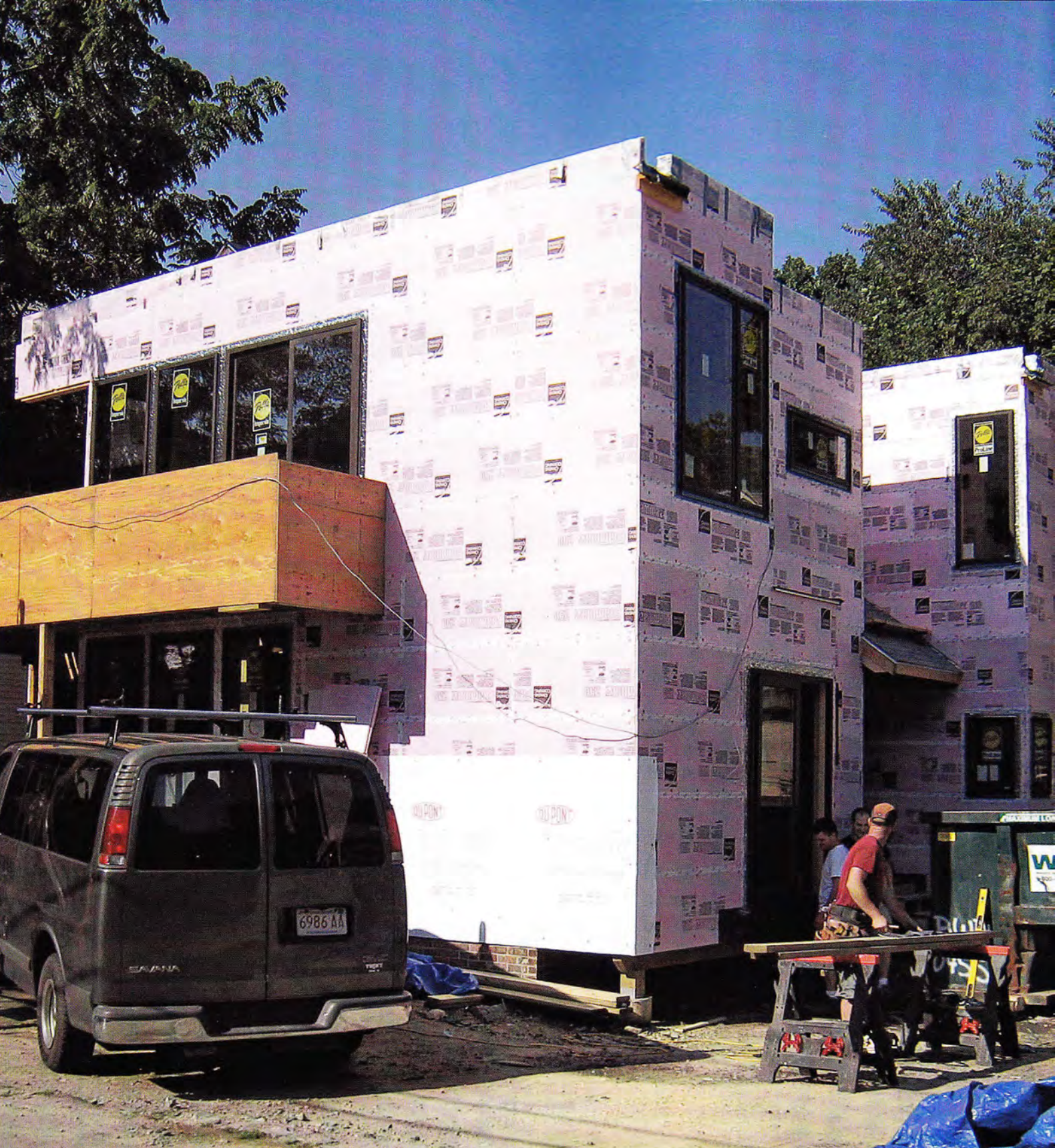
Improvements to the building envelope make a big difference in energy efficiency and should be a high priority for any green remodeling project.
